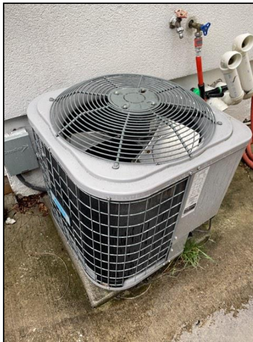
Air conditioner near the end of typical lif...
