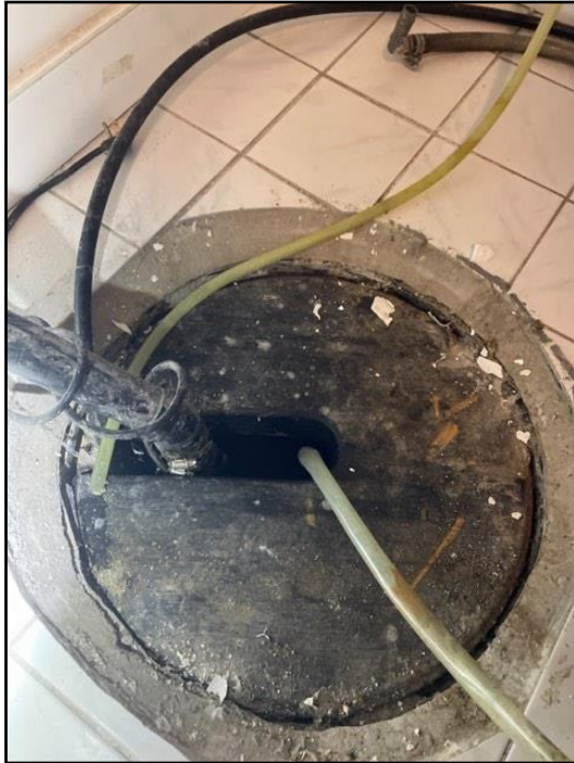
Sump pump was unplugged
