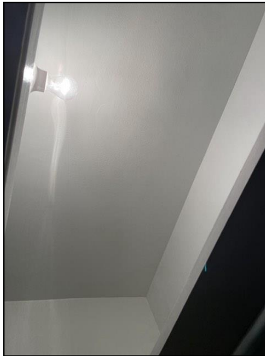
Improper closet lighting
