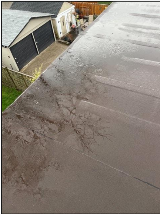
Water ponding on the roof
